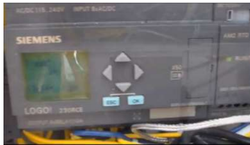
Figura IV.40. Logo 230 RCE Tablero de Control 50
